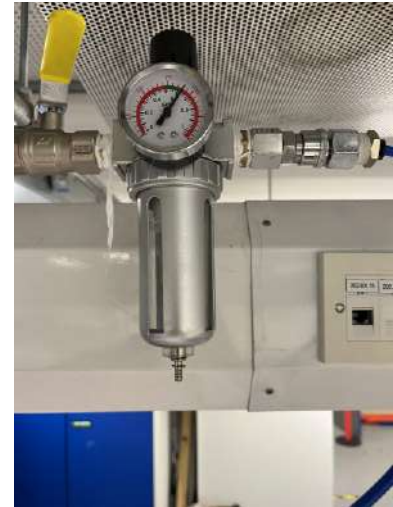
Figure 14: Compressed air gauge pump
